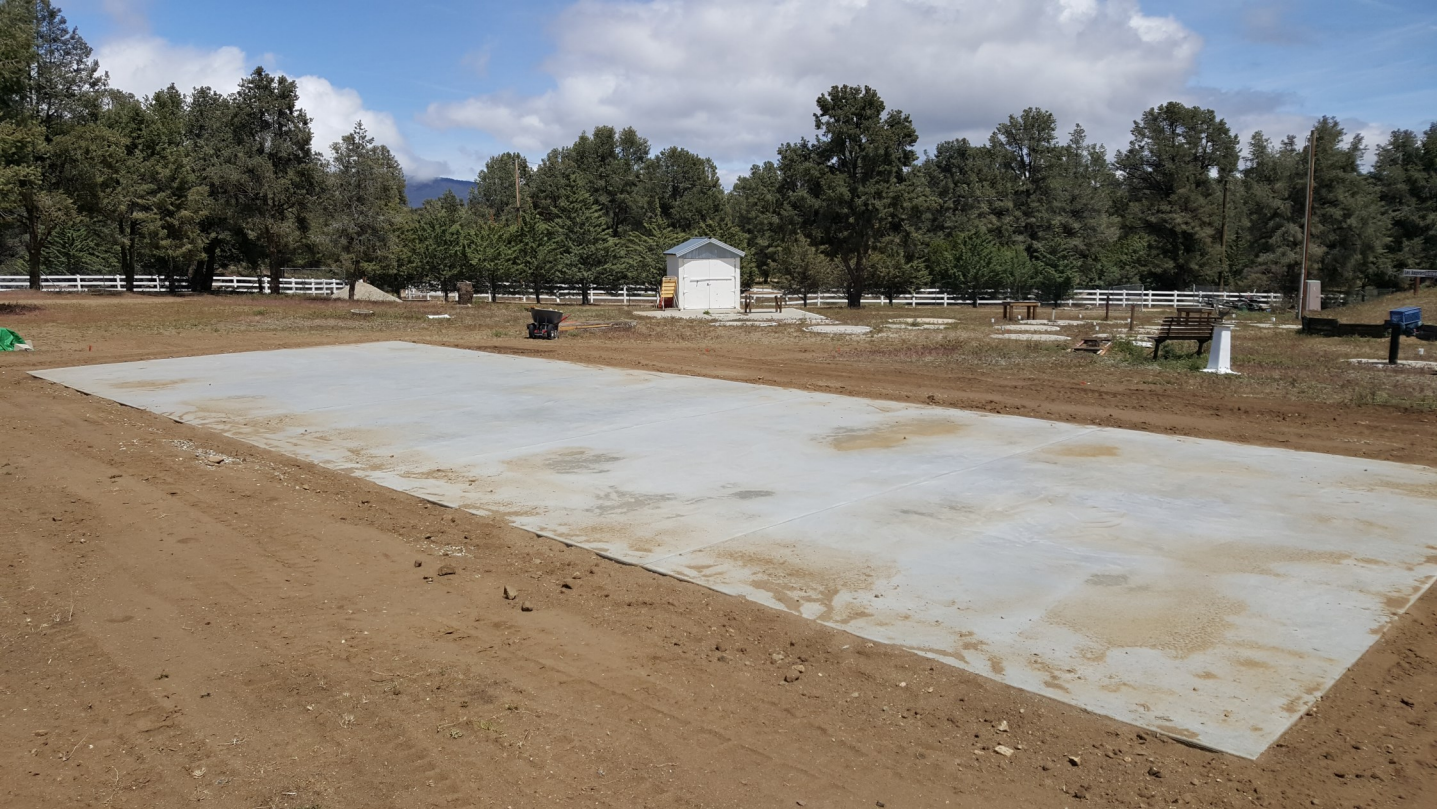
Here is a picture of the finished slab with some dirt from the rain. Photo credit: John O'Bryan, Jr.
