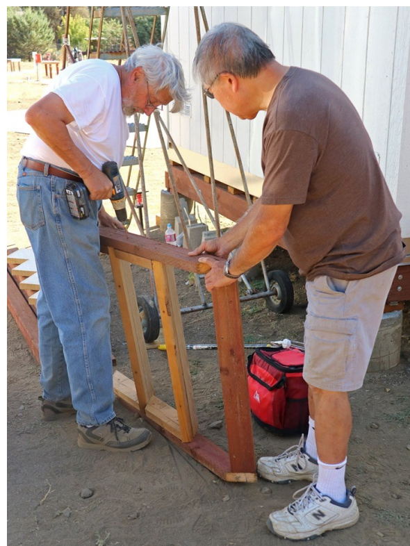
John O'Bryan and another member working hard on the new bathroom facility for the club. Photo credit: Ray Blumhorst
